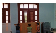
Fig. 1 — Trying to reduce the vulnerability of the premises associated with the ARES project using our own means.
